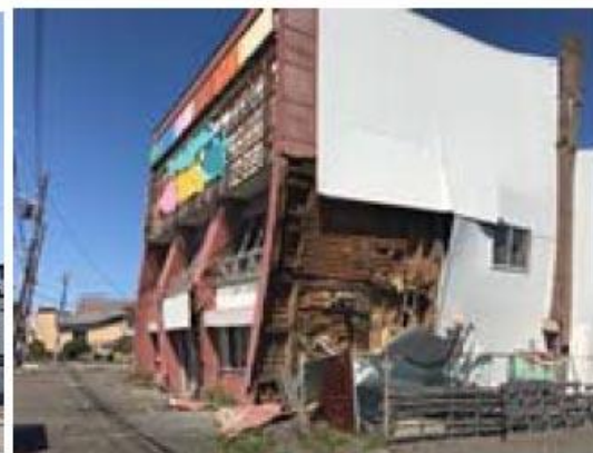
(c) 側面、壁の崩落
